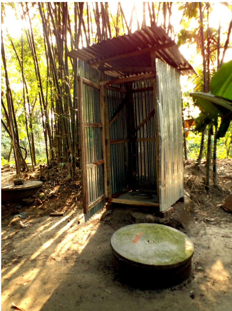
dual pit latrine
